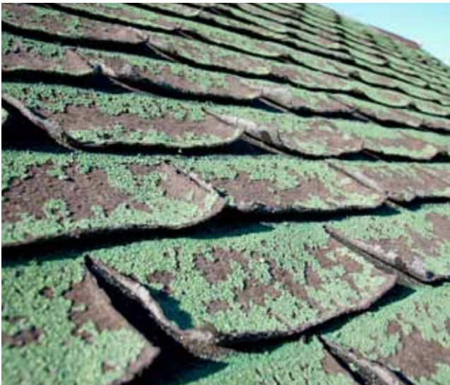
A poorly maintained roofing system past its economic life can result in costly building repairs beyond the cost of a new roof.
